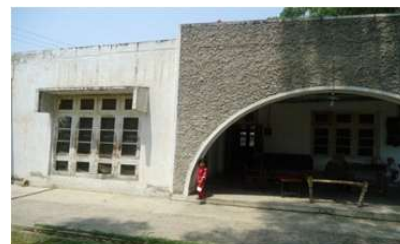
Basic Health Unit Before Repair
